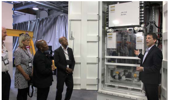
Representatives from South Africa's energy storage sector participate in a USTDA funded study tour with site visits in California.
